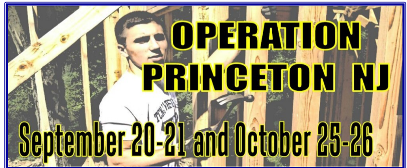
Altar server Anthony Cassar is working in what will become the Sanctuary of a new Orthodox Church in Princeton NJ. He is excited about serving in the new worship space! You can help make this dream a reality by supporting "Operation Princeton."
